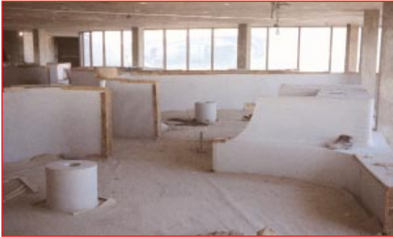
Flight Wing Two was actually the first to be completed, along with the original terminal construction. The ceramic-trimmed, cylindrical fixtures on the floor are ashtrays. (Alistair & Beverly Duncan)
